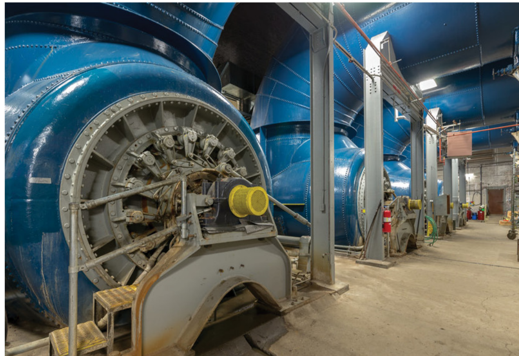
XCEL ENERGY ST. ANTHONY HYDROELECTRIC PLANT (VENUE LISTING ON PAGE 19)
